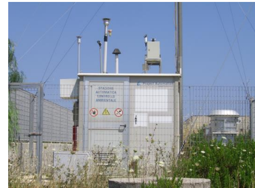
Monitoring local-site ARPA-PUGLIA: Air quality network, Brindisi Industrial Zone Brindisi, Italy
